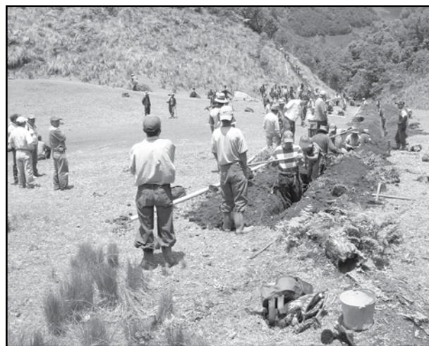
Community members in Cotzol, Guatemala, pitch in to dig a 5-mile water pipeline. Photo courtesy of Water For People.
