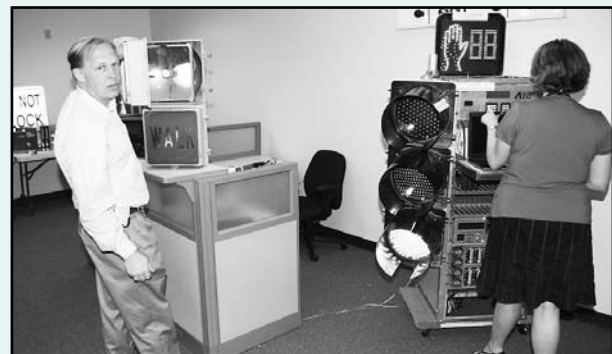
Traffic Services Manager Tom Udell shows off an "antique" pedestrian signal while Transportation Engineer Cindy Jenkins checks out a traffic signal control cabinet on display at Johns Creek City Hall.
