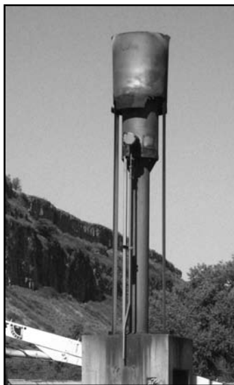
The old waste gas flare was in need of replacement.
