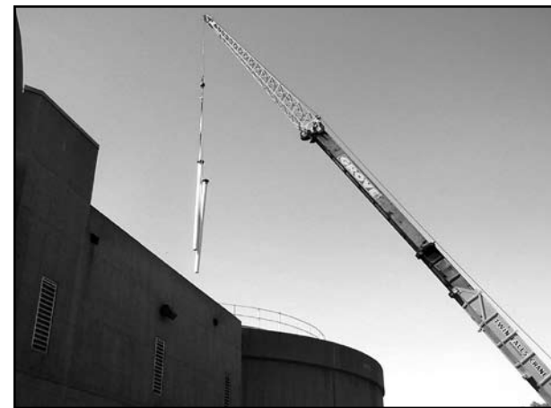
The crew used a crane to install the new piping in the digester.
