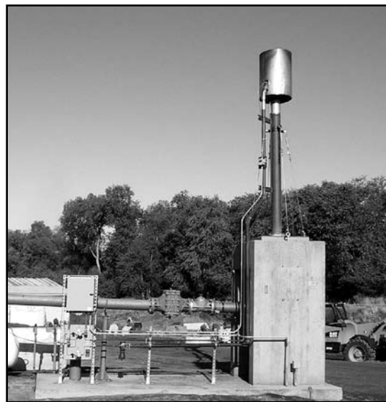
A view of the new flare that the Twin Falls maintenance crew installed.
